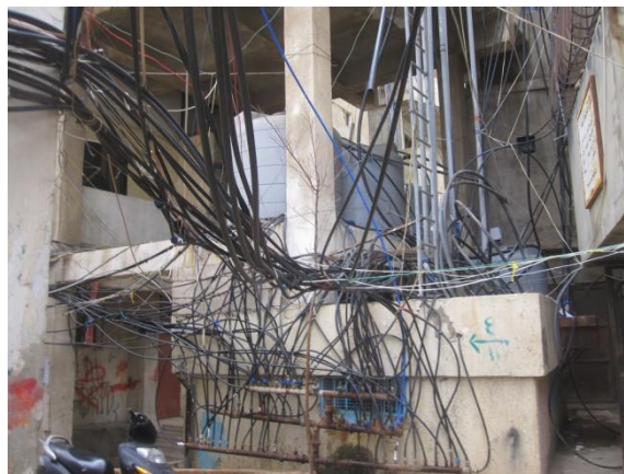
Figure 8. Tangle of wires in the improvised electricity system in central Beirut. Source: Emily O'Dell.
